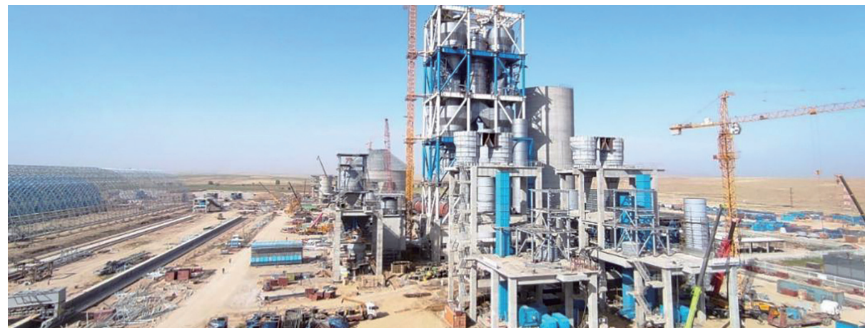
▲ The commissioning of 7500TPD clinker cement production line
