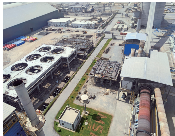
▲ Site of JSW waste heat power generation project
